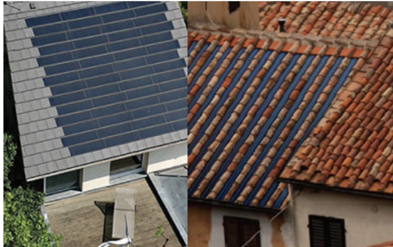
Figure 6: Examples of BIPV installation on roofs [24]
