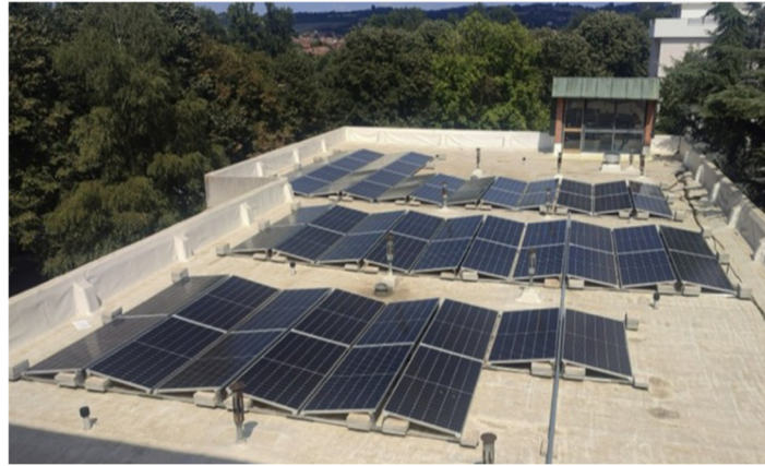
Figure 2: 30 kWp rooftop PV plant at the Faculty of Technical Sciences, Čačak
